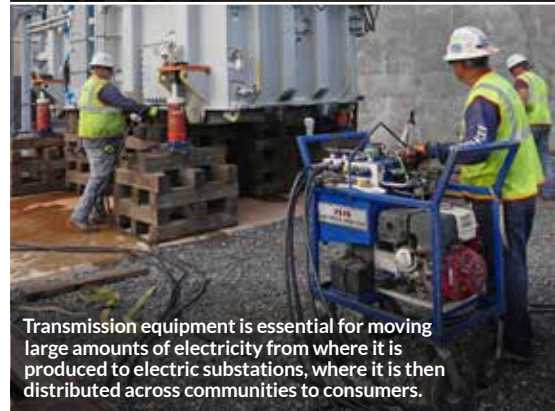
To keep pace with rising energy demand, new transmission equipment must be built, and existing equipment must be upgraded with the latest technology.
