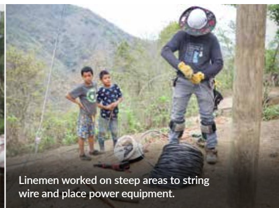
A villager checks out electrical equipment, which will power her home.
